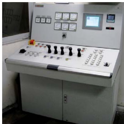
Figure 4: The new main control console.
