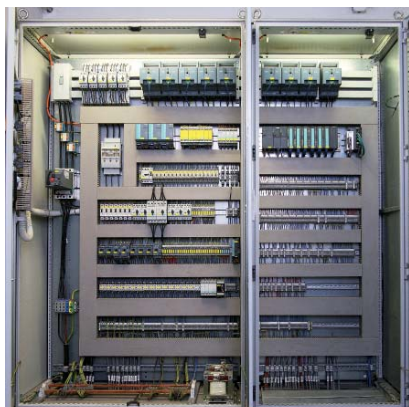
Figure 3: The new control cabinet.
