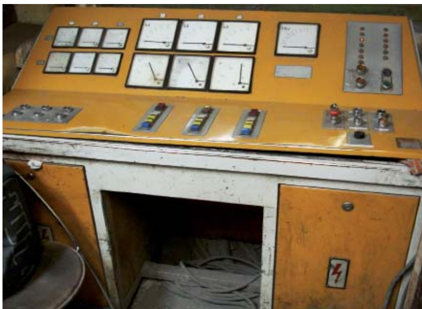
Figure 2: Operating control console – old design.
